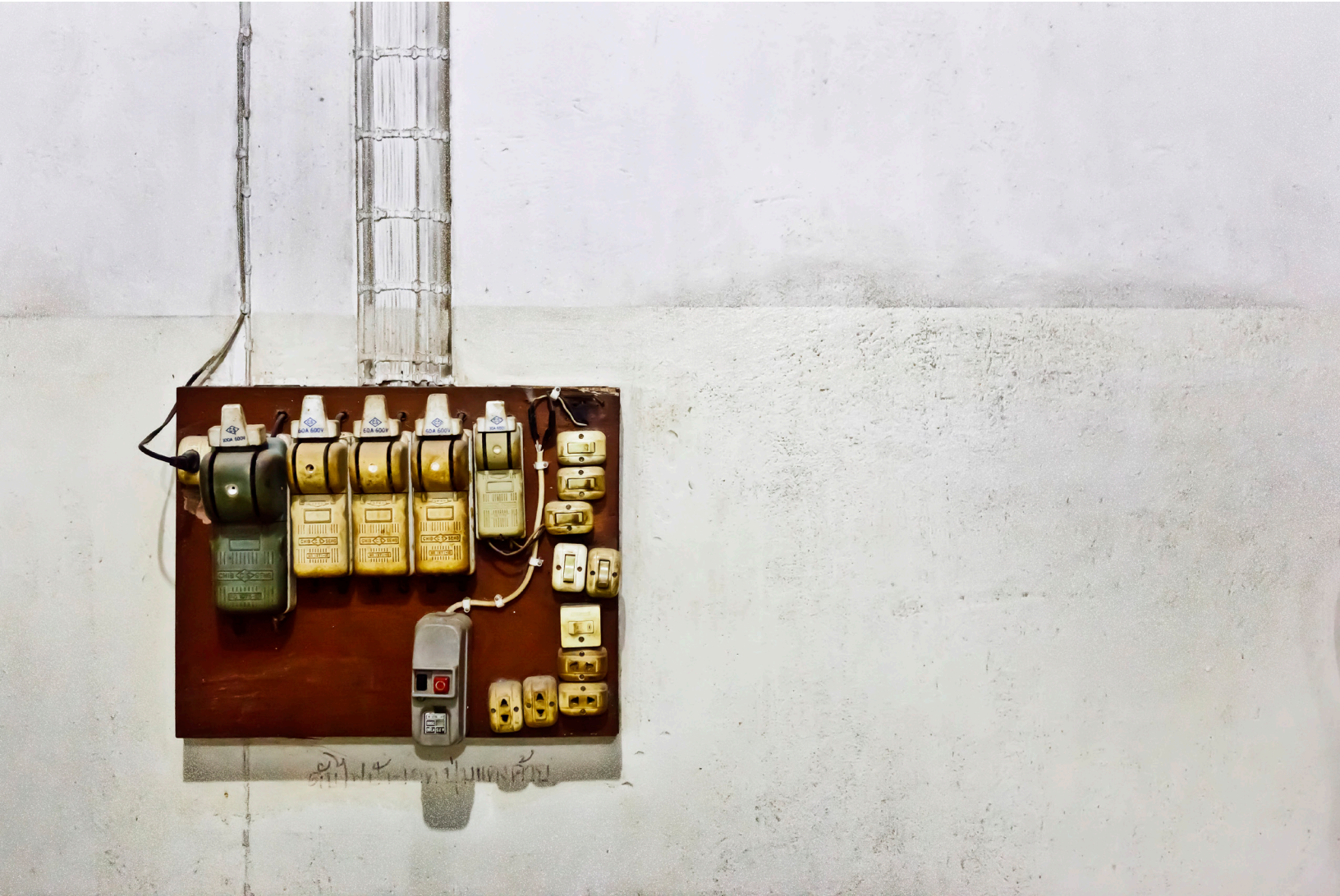
Fusebox and Switches. Uttaradit, Thailand
